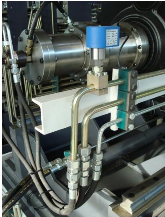
Picture 3: Leakage sensor fluid-Check with serv-Clip -2 for recognizing seal damages at cylinders of a reeling machine
